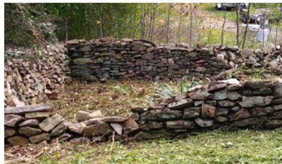
Fallen wall to be repaired
