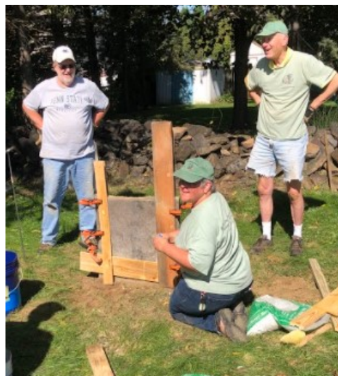
Marvin Stamm, Les Rohrbach and Lara Thomas repairing and righting a portion of a damaged stone at the Deturk/Rothermel burial ground.
