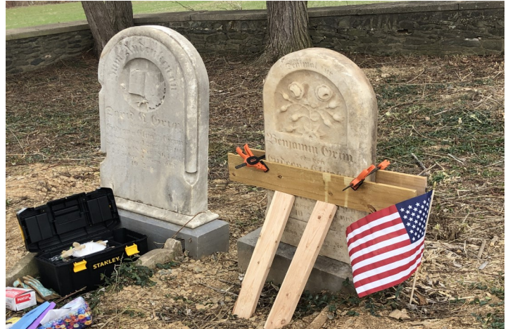
Repair work on Benjamin Grim (1797-1860) stone; a veteran of the War of 1812
